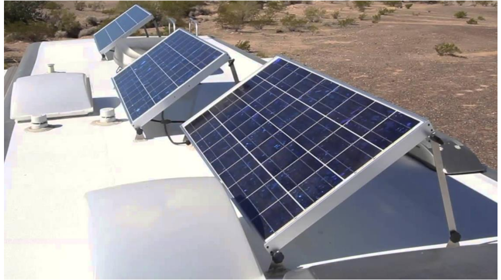
4x 250w PV Panels
